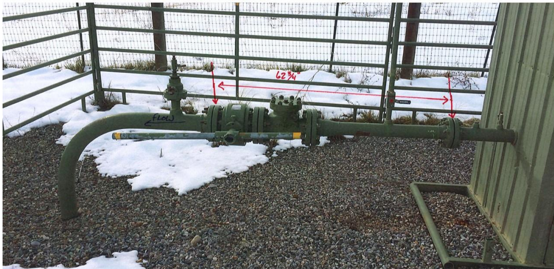
Figure 3: Removable spool at Pad 1 acting as launch site for EVO-Pig.
