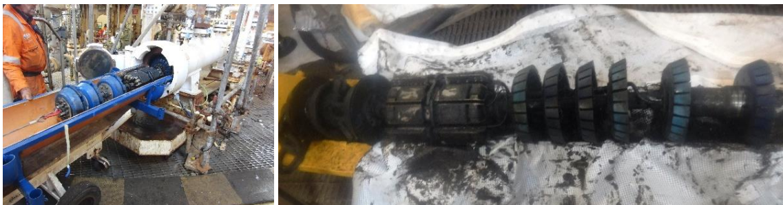
Figure 11-12: Receive of MFL inspection tool in 2013 (left) and 2019 (right)
