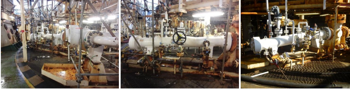
Figure 2-4: Launch / Receive area at turret
